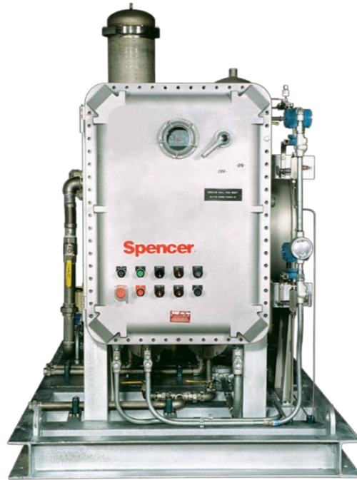
Control Panel featuring NEMA 7 enclosure controls the supply of bio-gas used as boiler fuel at a West Coast facility. It includes alarm and fault protection for high temperature and both low and high gas pressure.
